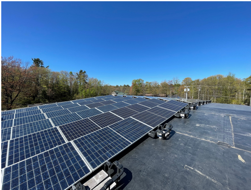
Negaunee Township Hall Solar System Installed by Peninsula Solar, 2022
